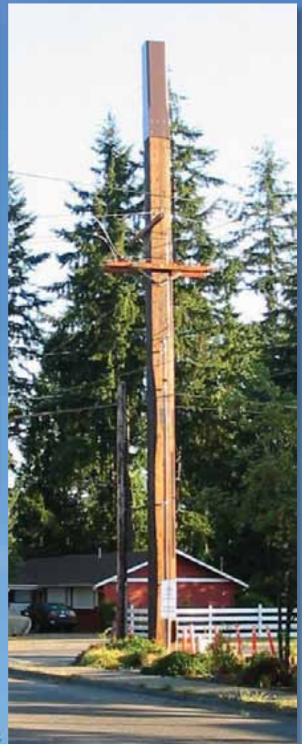
45' Distribution Structure with Concealed Antennas
