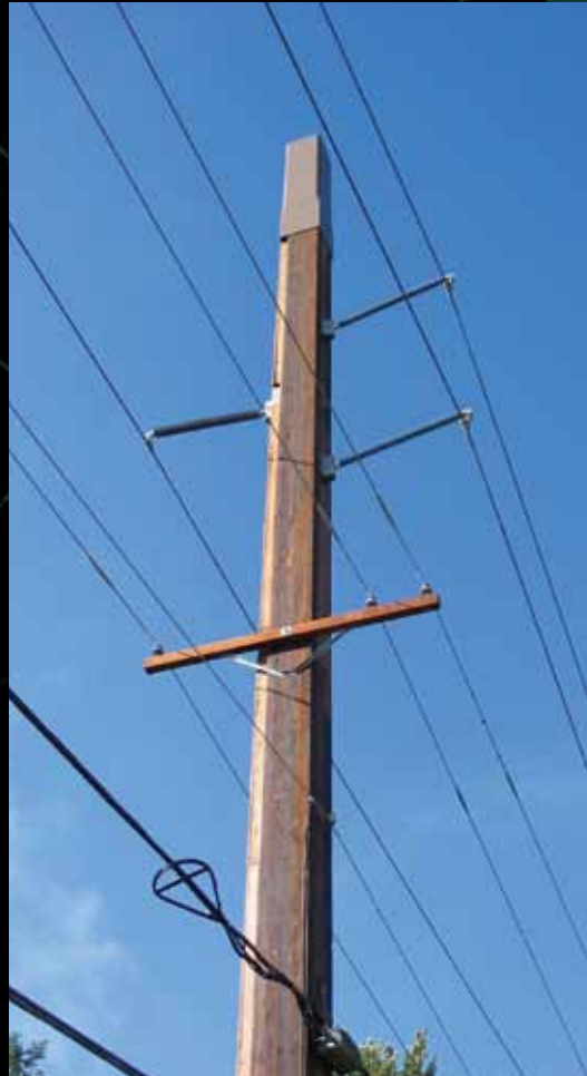
69' 115kV Transmission Structure with Distribution Underbuild, Cable TV Attachment and Concealed Antennas
