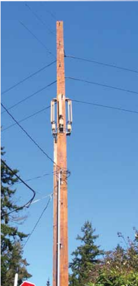
71' Distribution Structure with Flush-mounted Antennas
